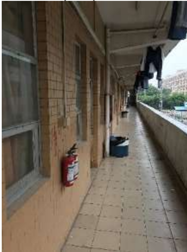
Dorm hallway is unobstructed
