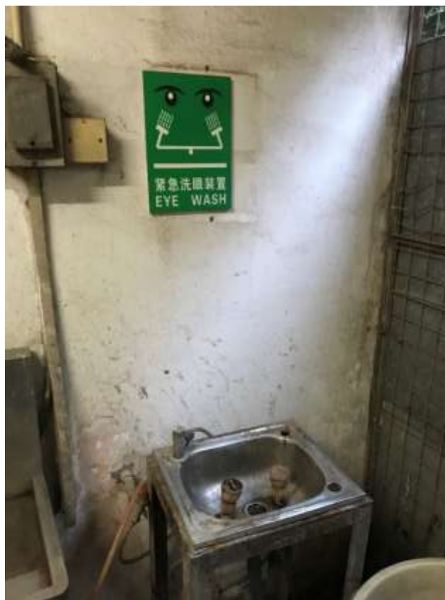
Emergency eyewash station
