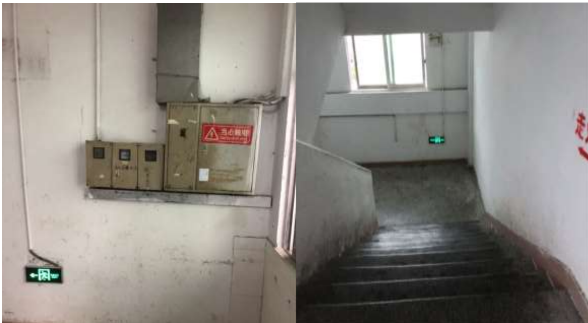
Emergency exit signs
