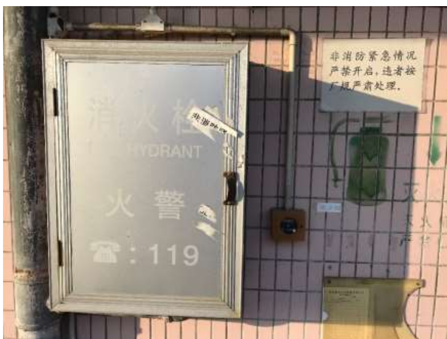
Fire extinguisher and fire hydrant
