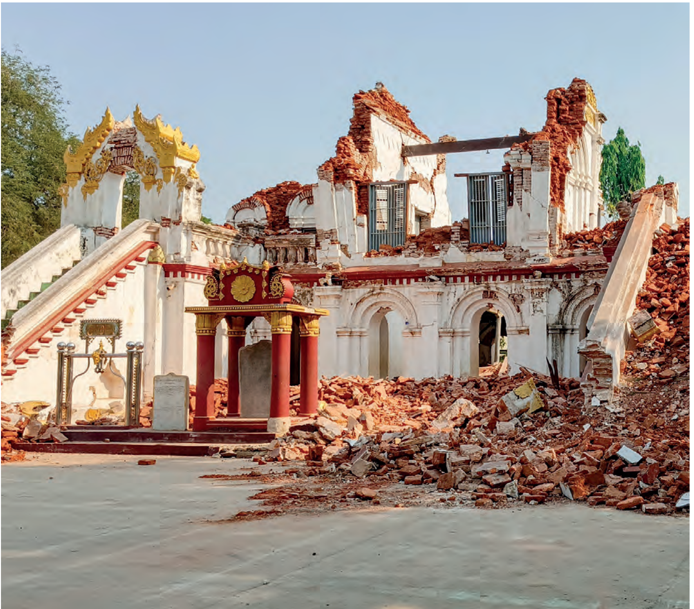
The severe earthquake in March 2025 left many houses in Myanmar either partially or completely destroyed.
